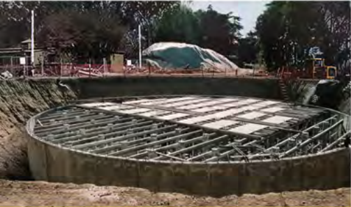
TreePeople Center Rainwater Cistern, Los Angeles, USA
