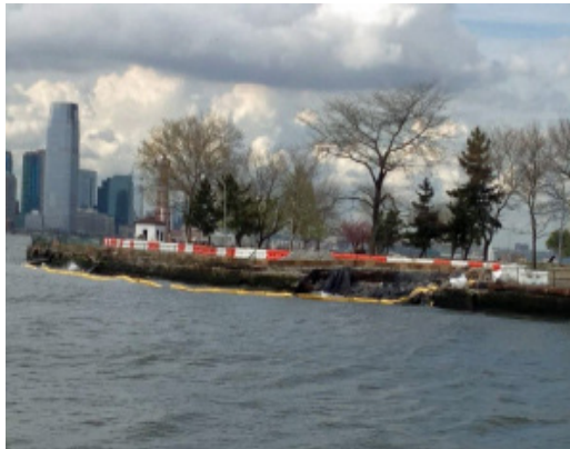
Kryton's Leak Repair System is able to withstand the constant water pressure the ocean puts on a seawall.
