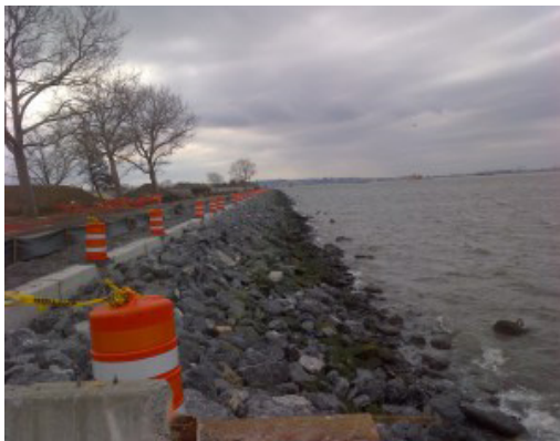
Over 2,000 yd3 (1,530 m3) of KIM concrete was used for the rehabilitation project.
